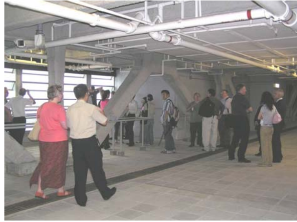
Figure 5 - Refuge floor in a Hong Kong high-rise during a fire drill Source: Arup (used with permission)
